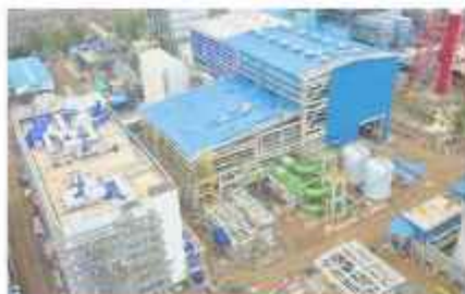
Power Plant 850 MW - Central Java
